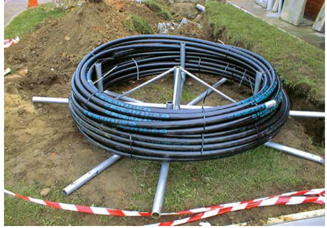
Fig. 2: A simple jig facilitates uncoiling of the flexible LPG piping on site.
