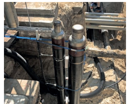
Proper securing and fastening of the connections
