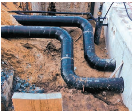
Connection of the technical center to the cooling line
